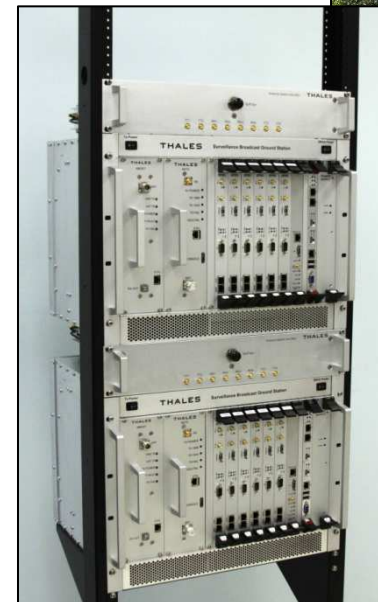
Dual redundant, quad channel, dual link SBS ground station
