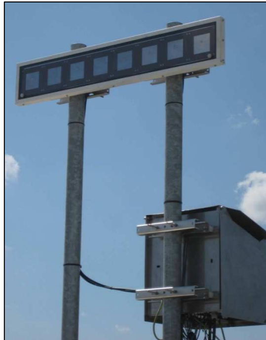
Antenna and Ground Station
